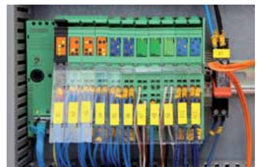
The ILC 150 ETH Inline controller and the connected I/O modules serve as a central unit for collecting all operating data.
